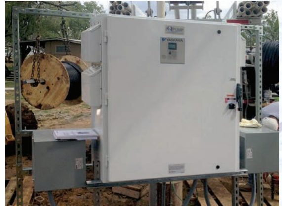
20 HP Submersible Pump Control for Irrigation.
